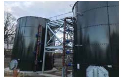
Above: New Sludge storage tank and external pipework. Below: Two new main sludge Pumps and pipework to the new Tanks.
